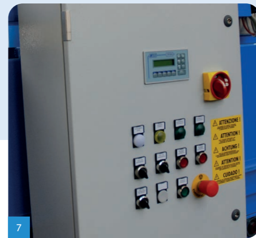
7 Control board and temperature management.
