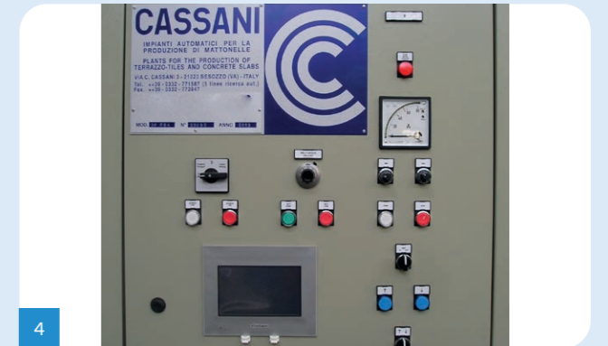
Control Panel with Proface.
