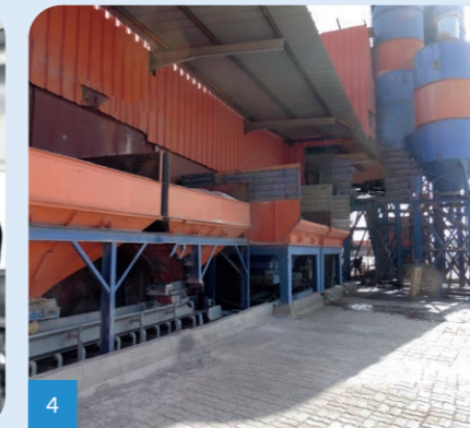
4 Exterior of plant with GR3A and cement silo.
