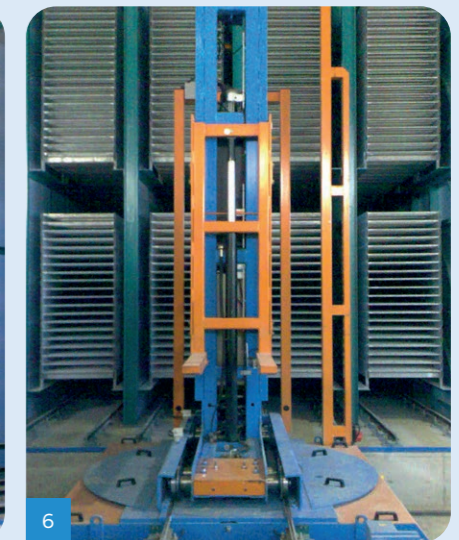
Robot trolley vertical loading of stack.
