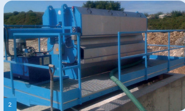
Filter 800 / 15 on platform.
