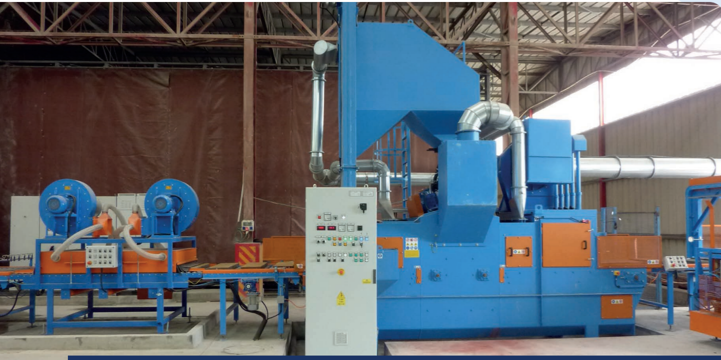
Drying machine leading to shotblaster.
