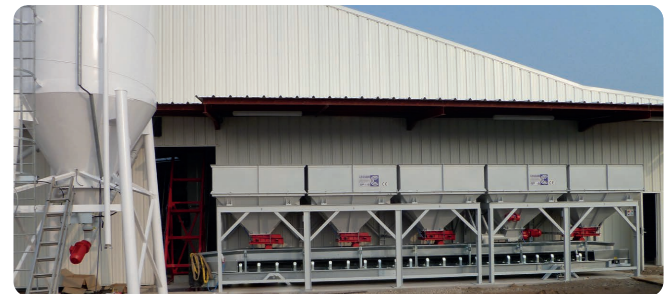
GR5A with weighing belt delivers material to the trolley for transportation up to the mixer platform (inside building).
