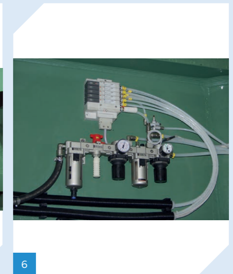
6 Pneumatic control unit.
